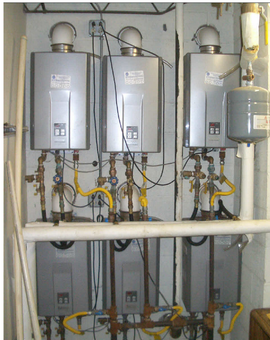
A bank of 6 Rinnai tankless water heaters
