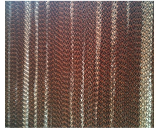
Evaporative cooling pad on June 25th, 2012
