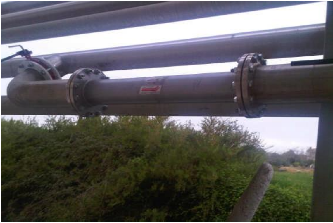
Picture of the 6" MagCAT Installed at Alier Papel
