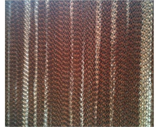
Evaporative cooling pad on June 25th, 2012
