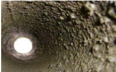
Feed Line to compressors with scale deposition
