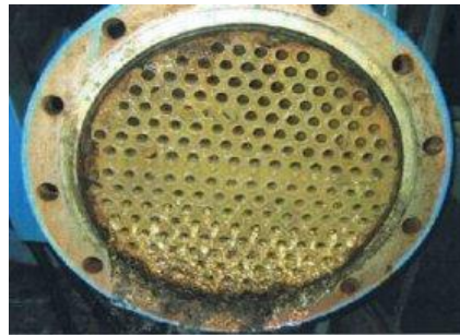
Compressor after cooler with scale
