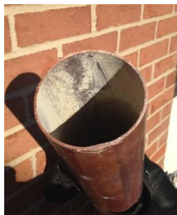
Scale in 3" Copper Feed Pipe
